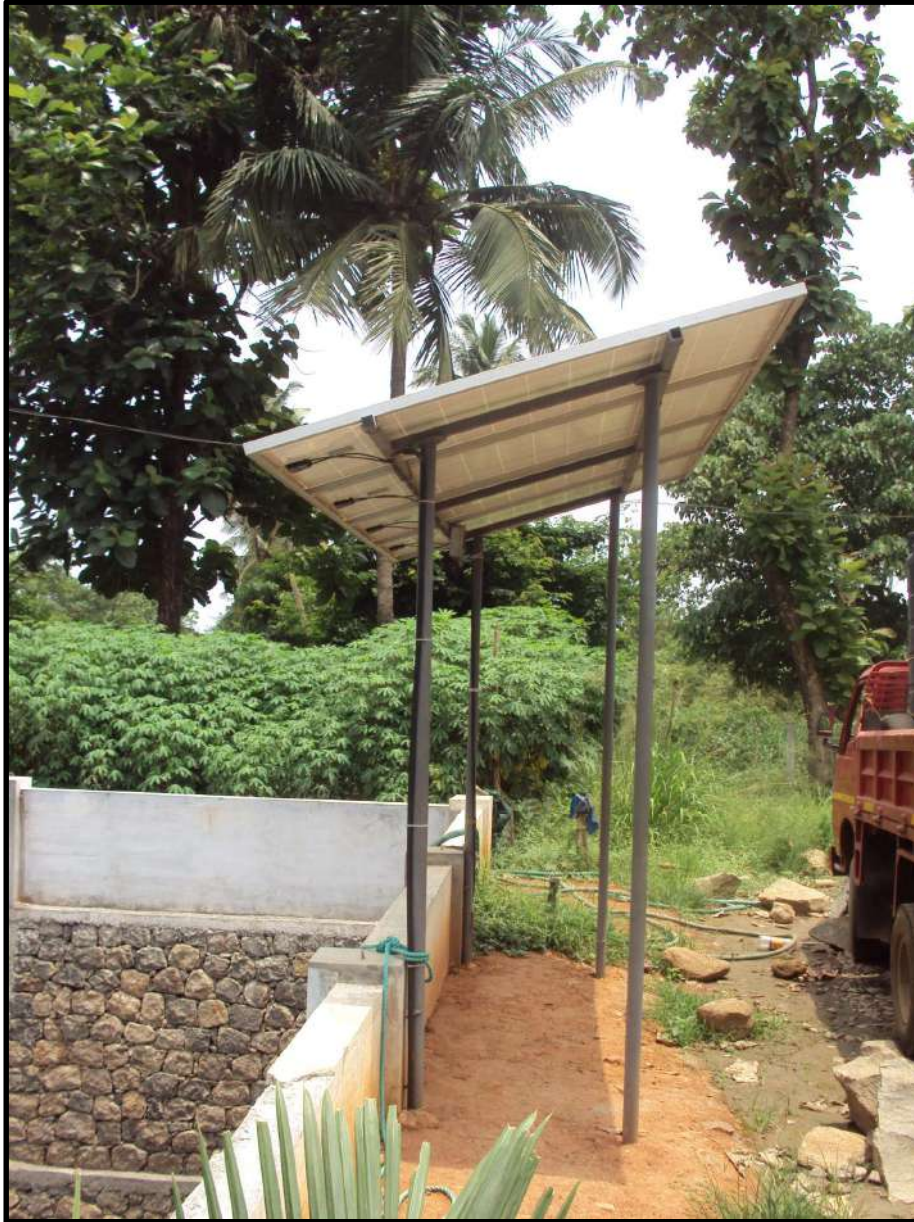
Photograph showing solar panel installed in the project area
