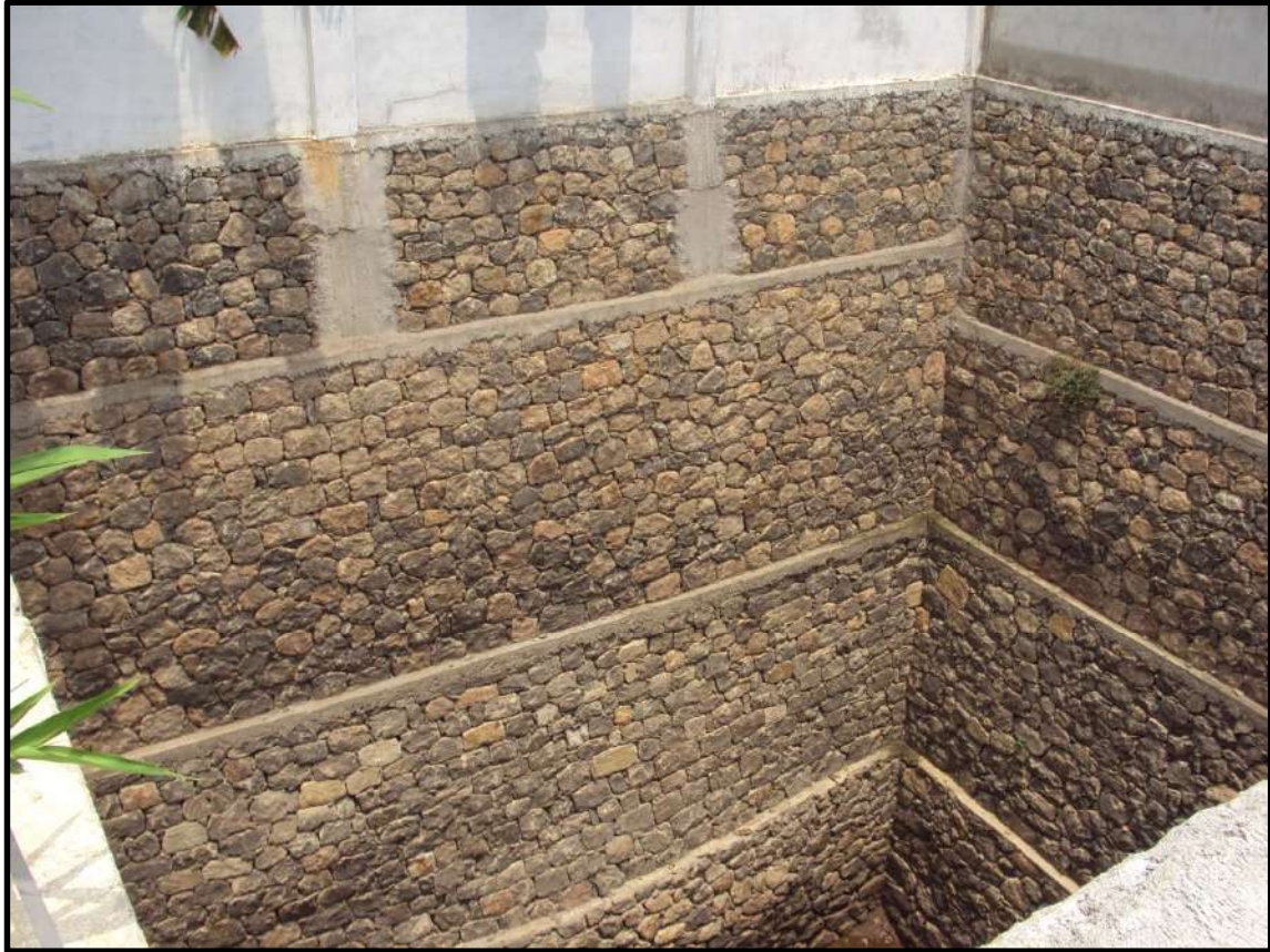
Photograph showing the rain water harvesting tank
